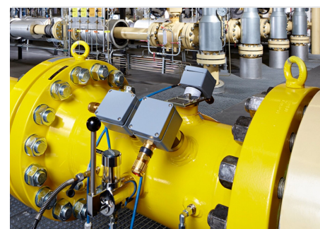
SM-RI-X at Pigsar HP calibration facility
